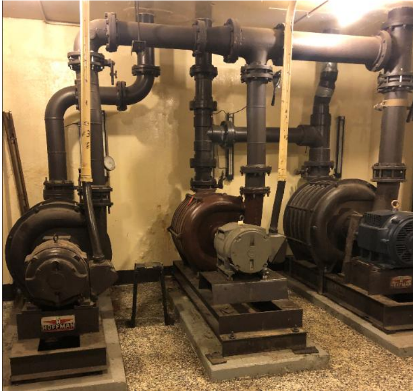
Figure 2-9 Aeration Basin Blowers
