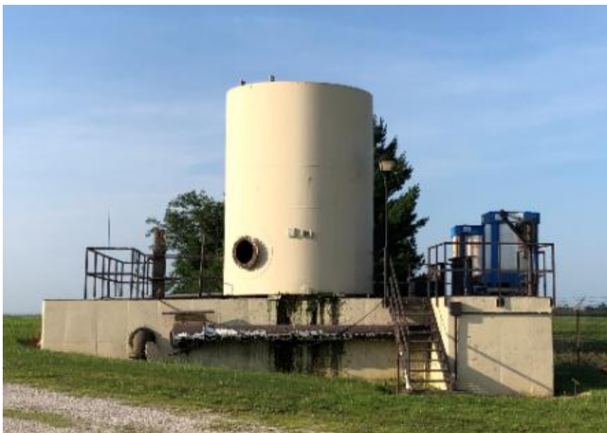
Figure 2-7 Primary Clarifier and Roughing Filter Recommended upgrades are:
